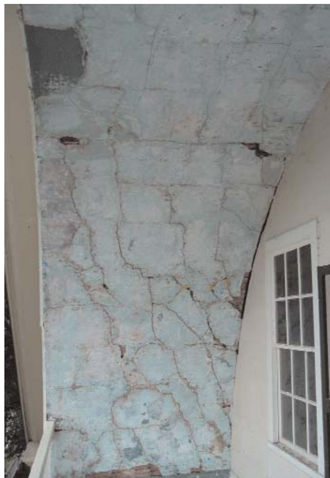
The inappropriate materials, including a moisture-trapping paint, used on the third-story porch of this Grafton, VT, house lead to peeling and cracking paint and plaster. Here, the paint has been removed to expose the plaster problems.
