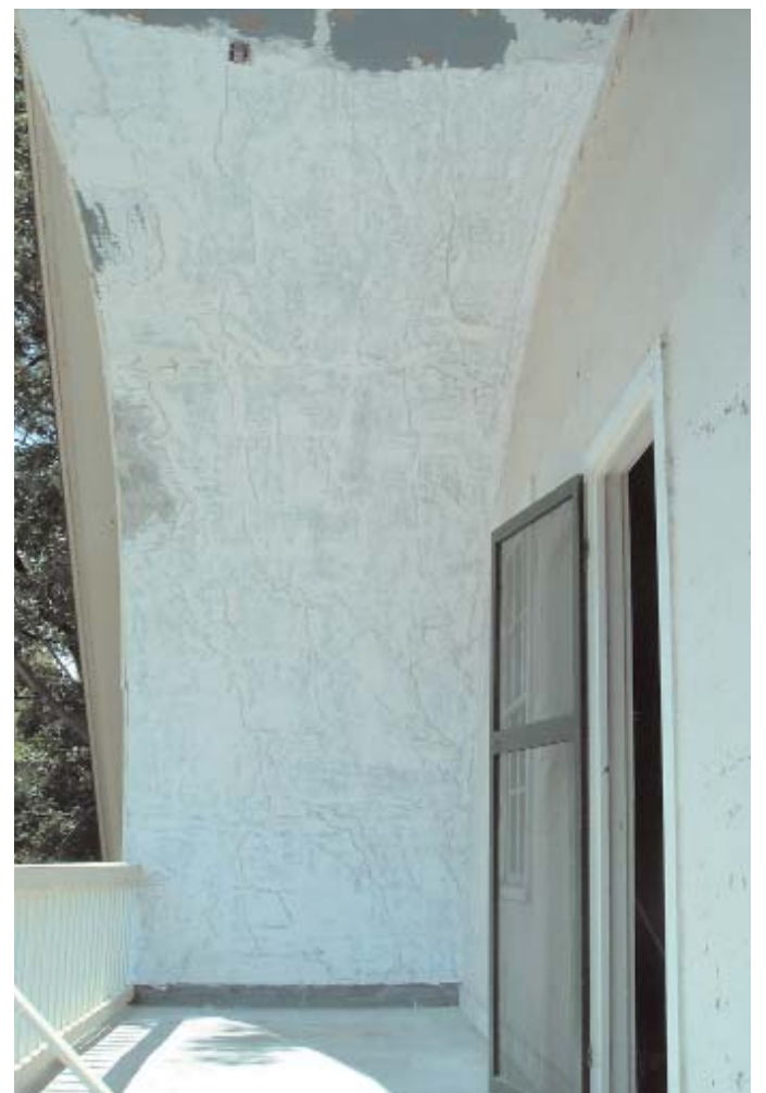
Brennan salvaged the maximum amount of plaster possible. The completed repair features skimmed and faired surfaces, which are now prepared for decorative painting.
